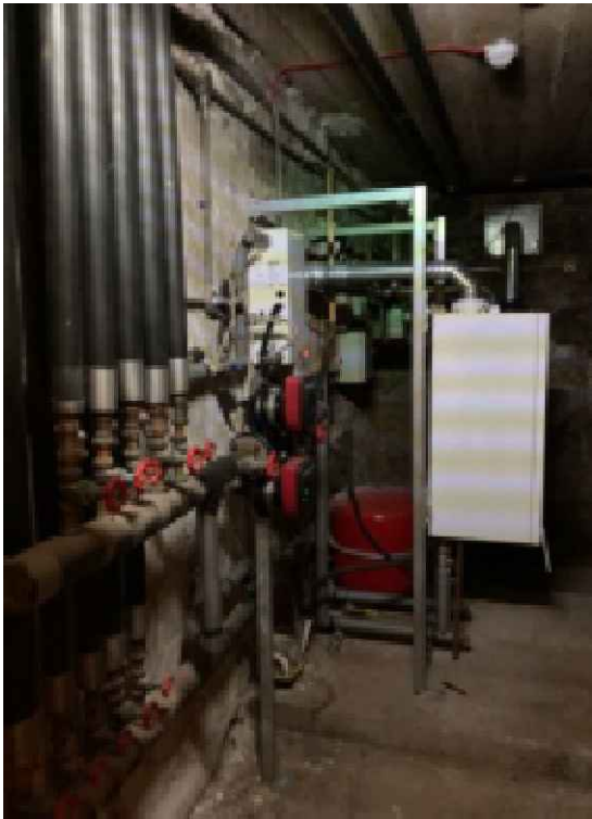
0 IMAGE REF 8 - BOILER ROOM Scale: NOT TO SCALE
