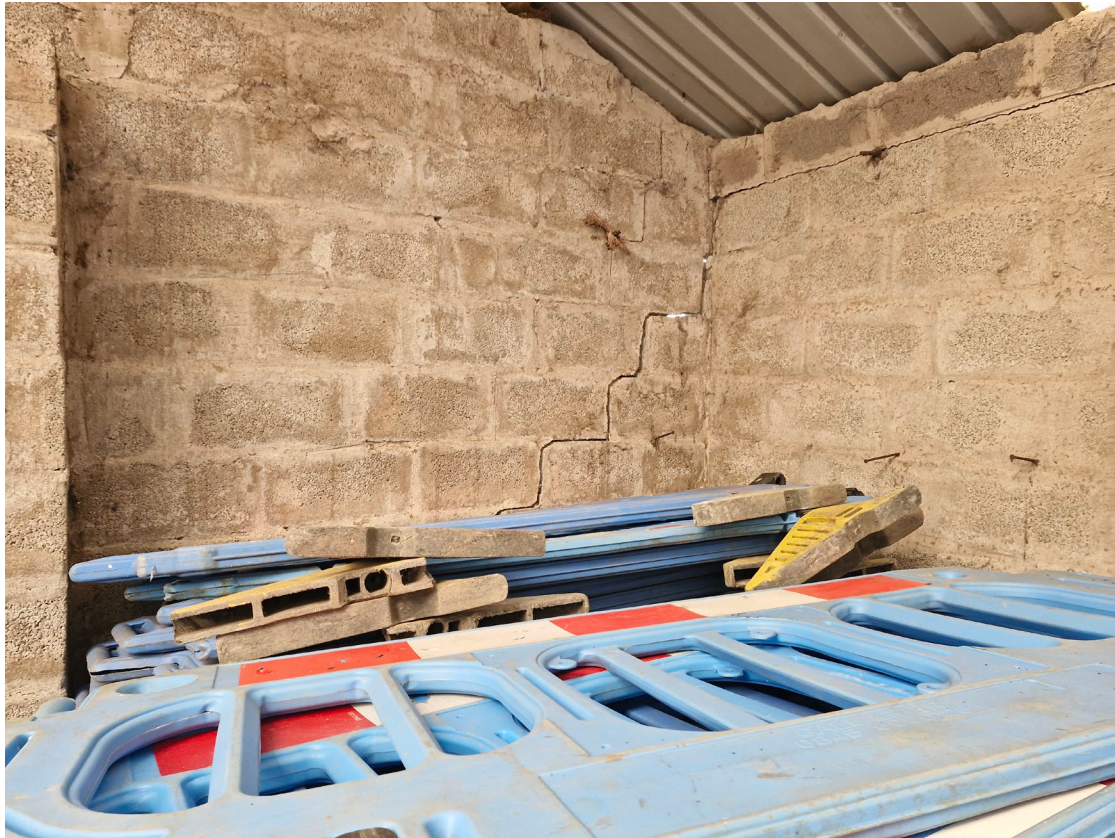
PHOTO 09 CRACKING TO REAR WALL BARN 4
