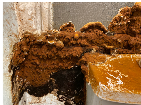
Enlarged image of dry rot.
