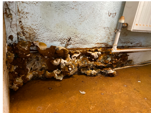
Image of dry rot at low level, above the suspended timber floor structure.
