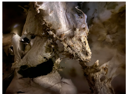
Image of dry rot below the ground floor level, within the sub-floor void.
