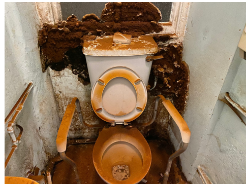
Image of the W.c within the two storey extension and the extent of the dry rot found therein.
