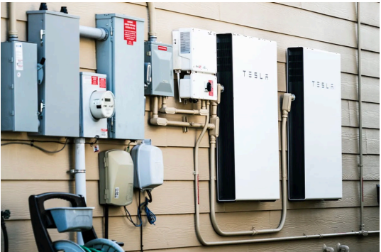
Typical solar panel equipment and batteries
