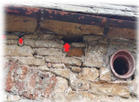
Plate 6: Gaps at wallhead.
