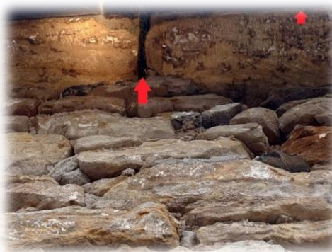
Plate 5: Gaps at wallhead.
