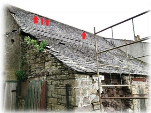
Plate 2: Gaps at ridge (SE aspect)
