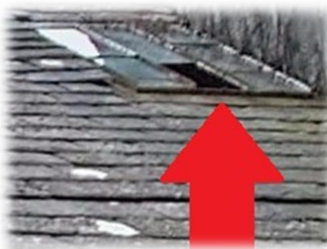
Plate 9: Gap in broken skylight window (SE aspect).
