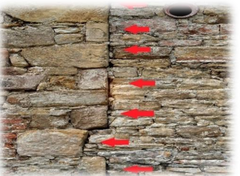
Plate 8: Cracks in wall SW aspect).
