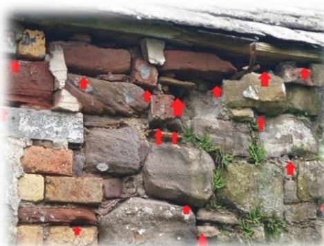
Plate 7: Gaps in mortar.
