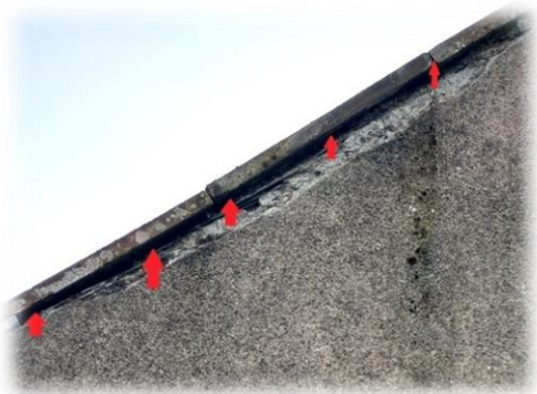
Plate 4: Gaps under coping stones.
