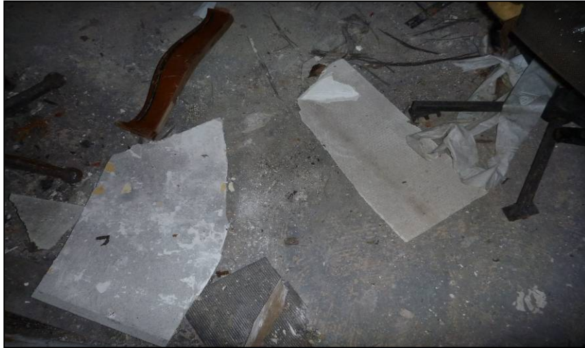
Photo 7: Asbestos insulation board waste in building
