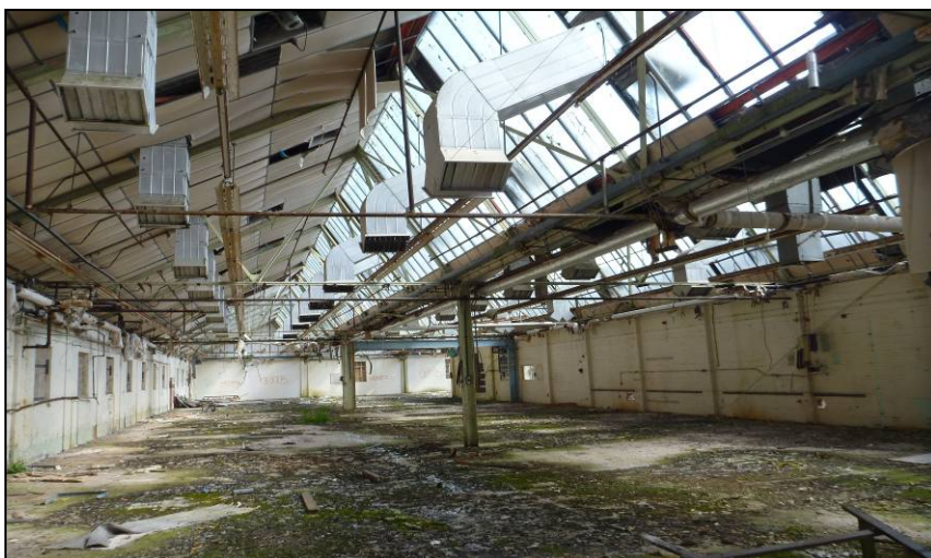
Photo 6: Interior of 1960s addition, to northwest of older building with cement roof and debris
