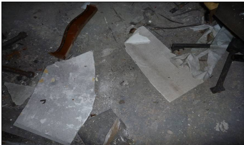
Photo 7: Asbestos insulation board waste in building
