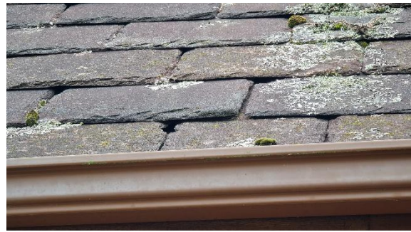
Photo 8: gaps and crevices a plenty
