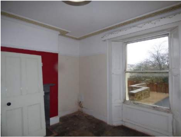
Left: Existing lounge architraves, cornices, and skirtings to be retained and repaired where hairline cracks have appeared.
