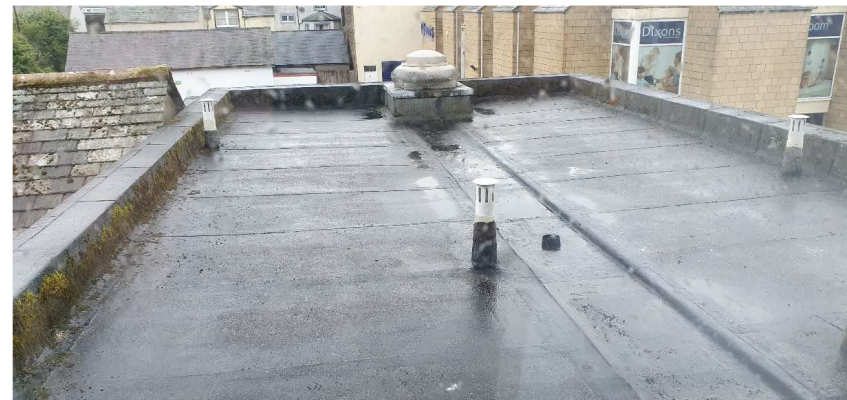
Flat roof damage with redundant M&E equipment
