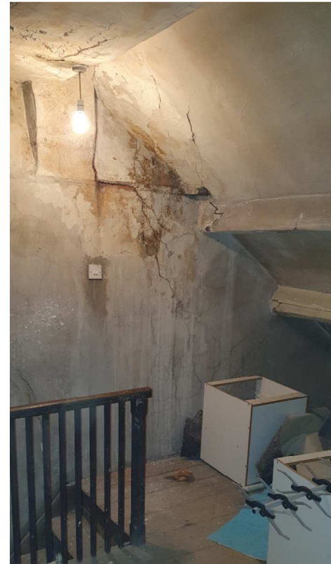
Water Ingress – within loft to be converted.
