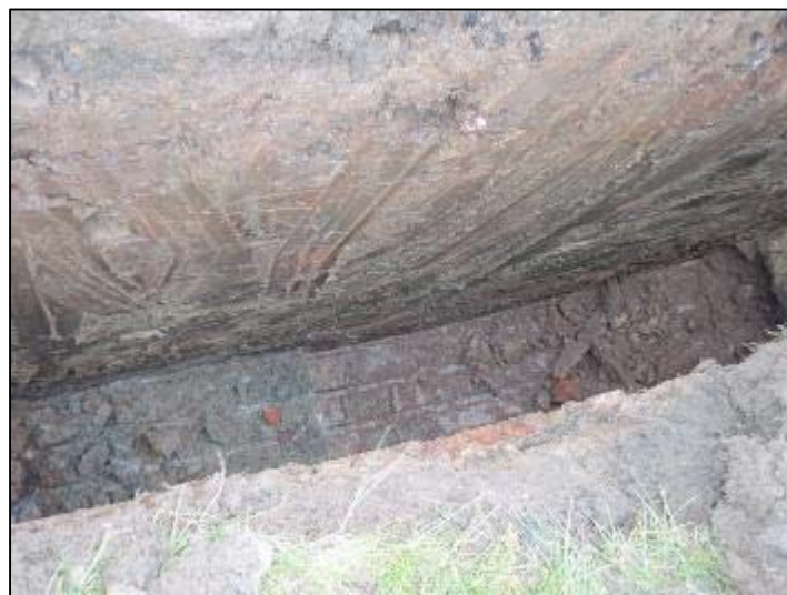
Photo 9: TP2 exposed boundary between the grey shale opencast backfill on the left with the red / brown natural clay on the right.
