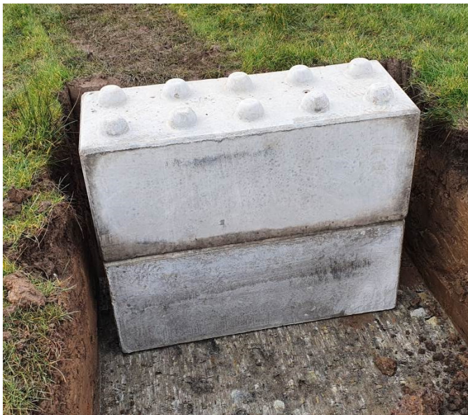
Figure 1: Blocks stacked directly on backfill
