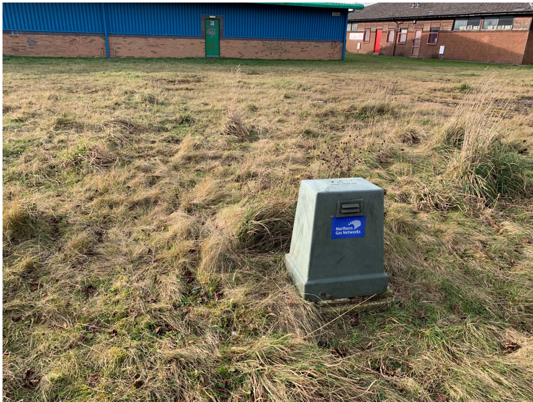
Photo Plate No. 05: Gas service marker in east behind parcel depot.
