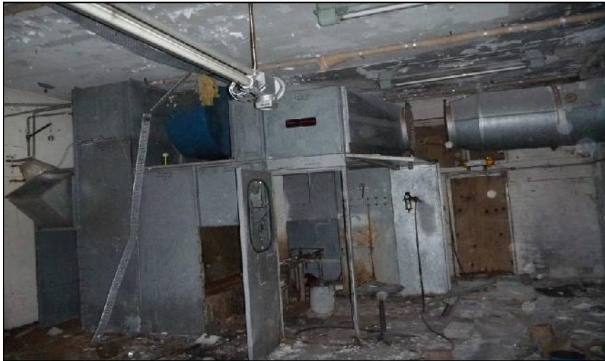
Photo 8: Glue cabinet in older section of mill building
