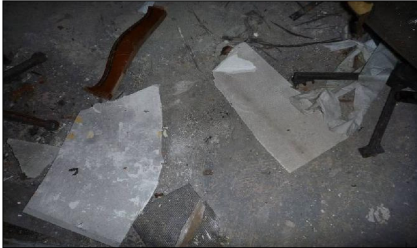
Photo 7: Asbestos insulation board waste in building
