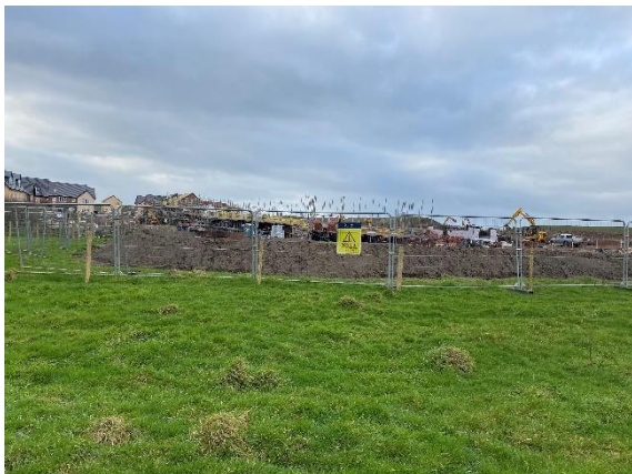
Photograph 16 – Area of construction site encroachment
