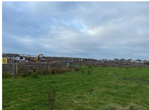
Photograph 17 – Area of construction site encroachment
