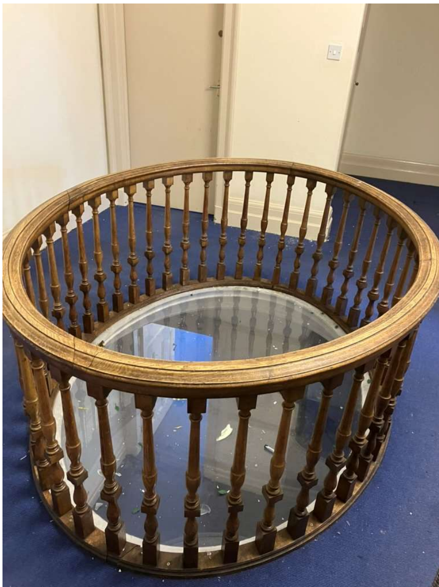
Internal feature between floors, Perspex infill to be replaced with fire resistant structure
