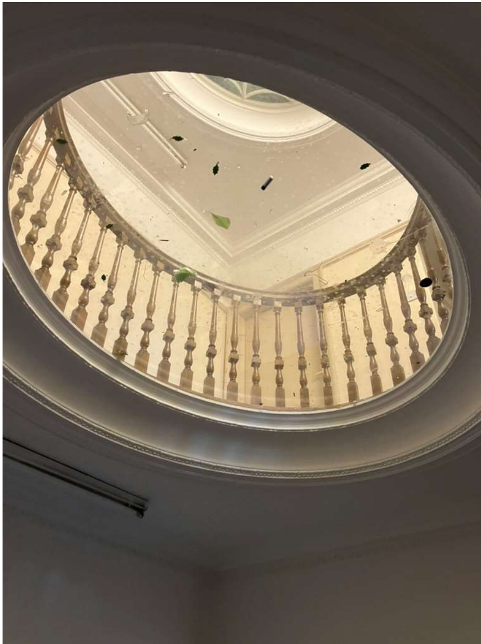
View from first floor with corresponding glazing in second floor ceiling – glass in roof position is now damaged
