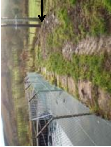
Flood crest Upstream (rutting)
