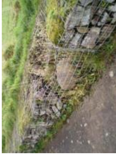
Gabions in Very Poor condition (Grade 5)
