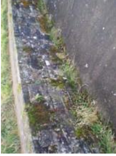
Minor grass growth in masonry wall joints
