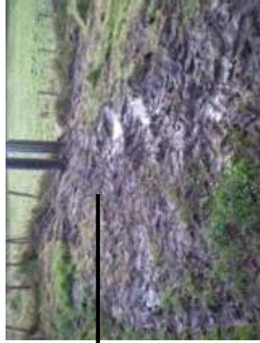
Outward face and Flood crest (heavy poaching)
