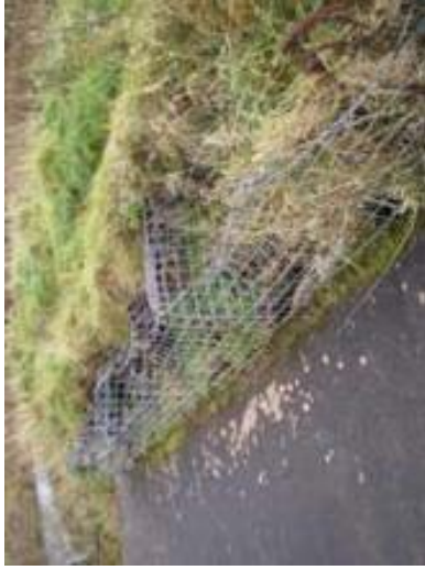
D/S gabion baskets in failed condition
