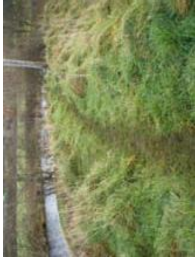
Crest heavily vegetated with rutting
