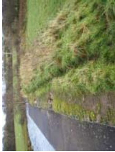
Heavily overgrown flood crest
