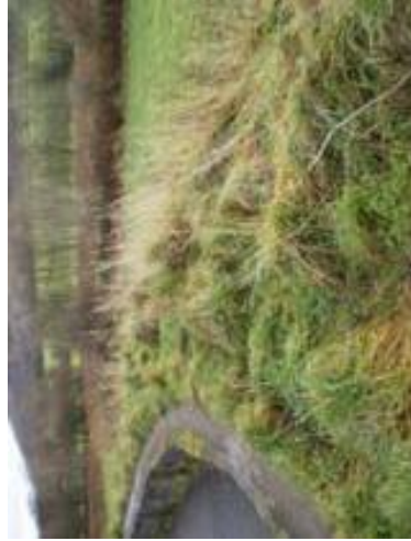
Heavily overgrown Flood crest
