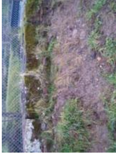
Heavily eroded outward face
