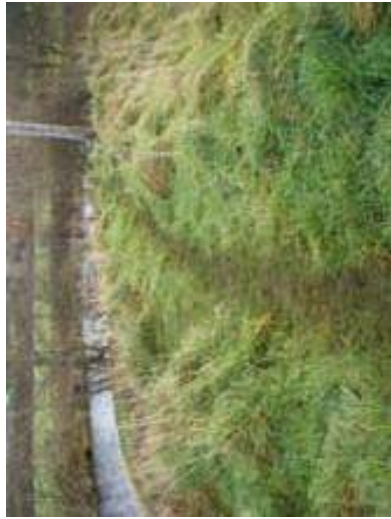
Crest heavily vegetated with rutting
