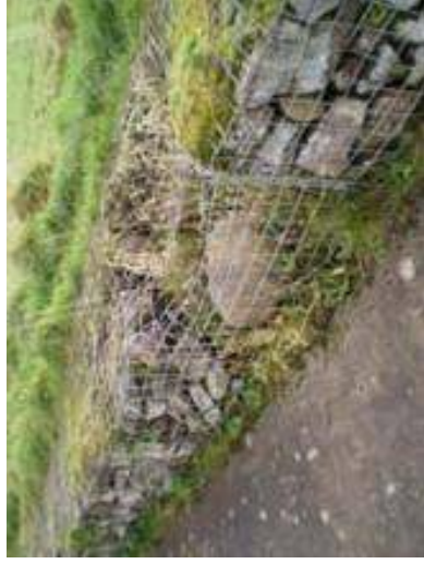
Gabions in Very Poor condition (Grade 5)
