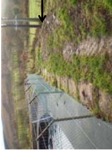
Flood crest Upstream (rutting)
