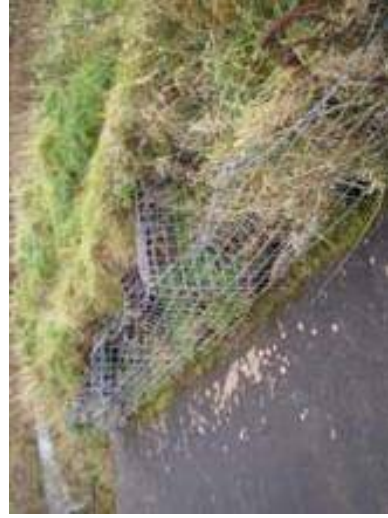
D/S gabion baskets in failed condition
