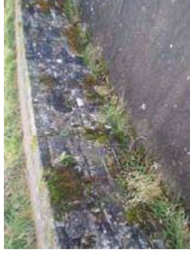
Minor grass growth in masonry wall joints
