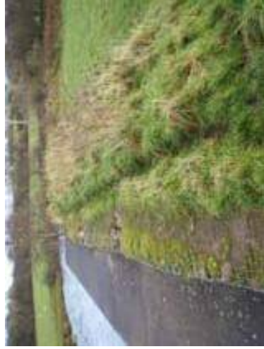
Heavily overgrown flood crest
