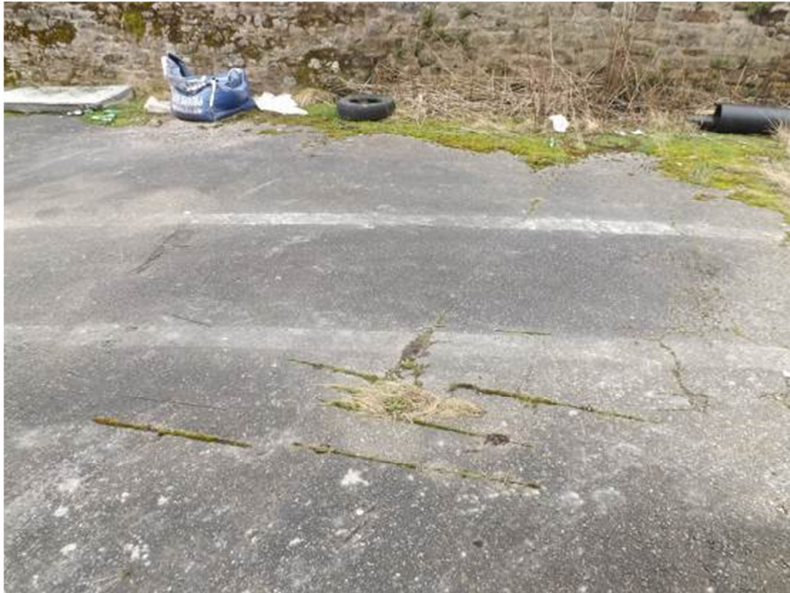
PLATE 7 – AREA OF SURFACE SUBSIDENCE IN SOUTHERN AREA OF SITE
