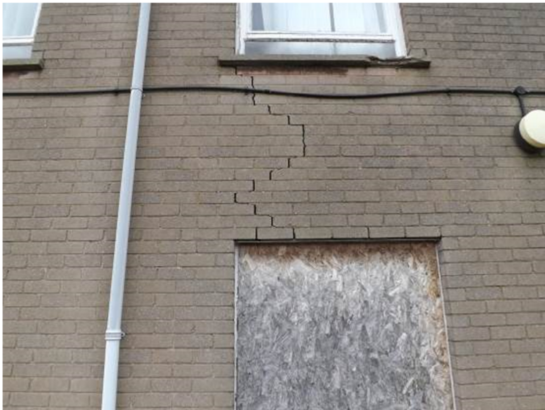
PLATE 6 – VERTICAL CRACK TOP TO BOTTOM OF OFFICE BUILDING
