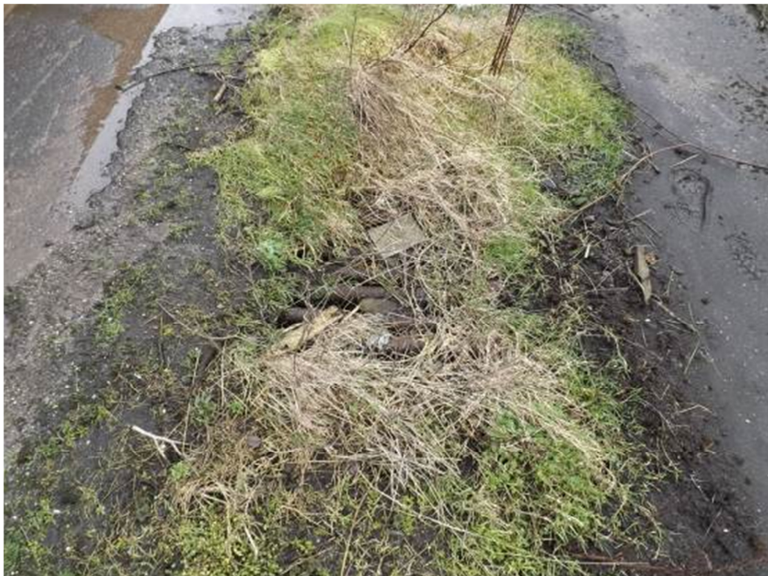
PLATE 8 – DRAINAGE GRID/INTERCEPTOR IN SOUTHERN AREA OF SITE CLOSE TO CP103
