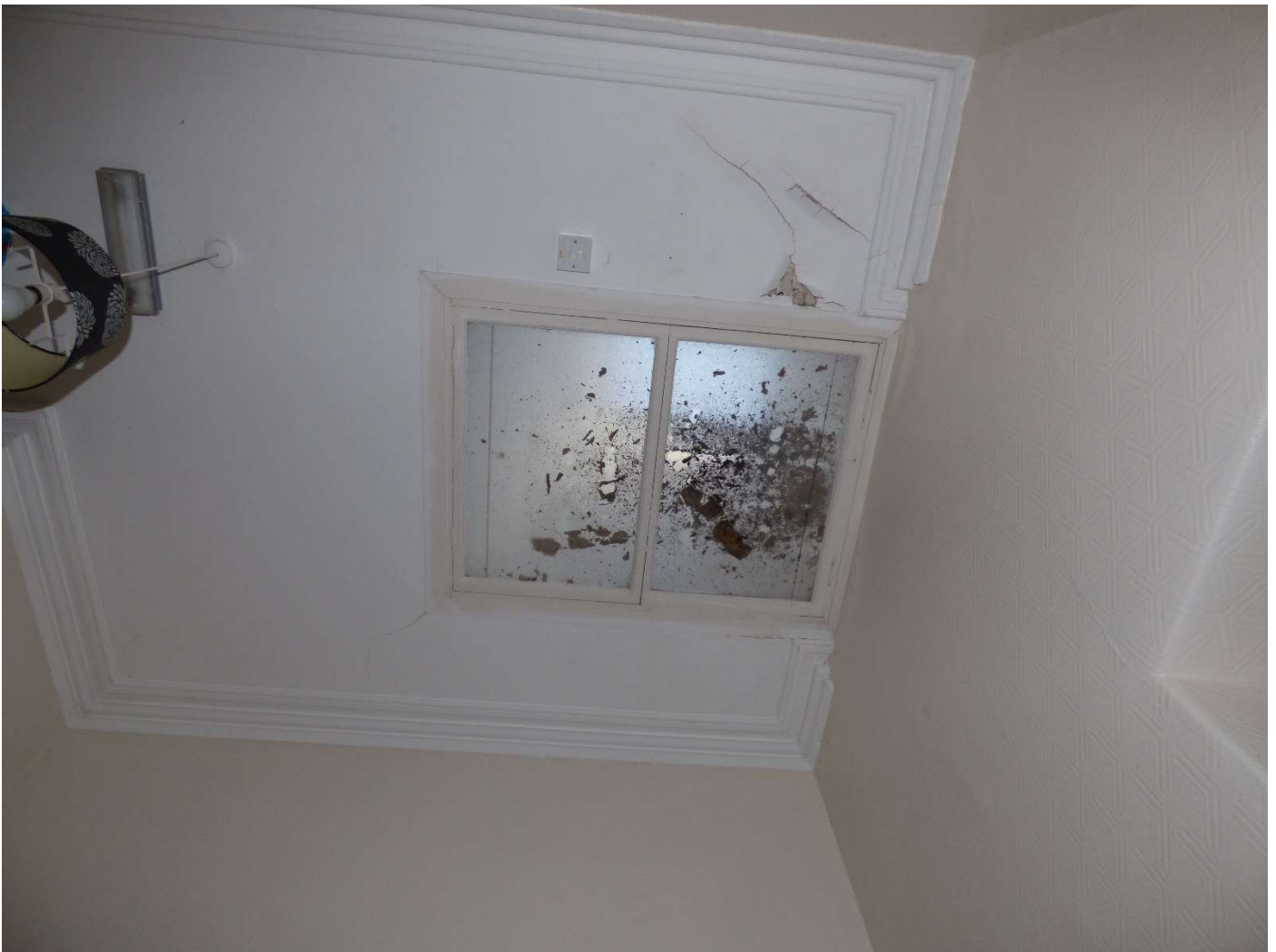
Above: House 7 ceiling light.
