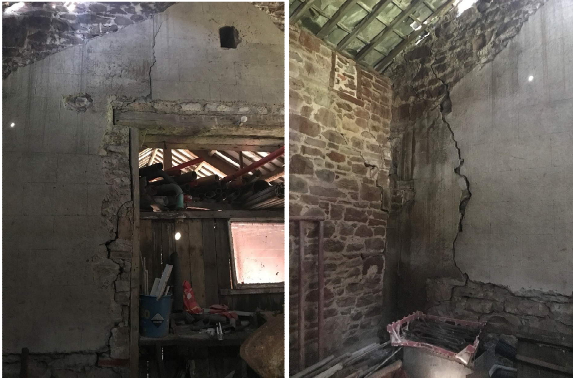
Figure 3.12 – Cracking in internal wall
