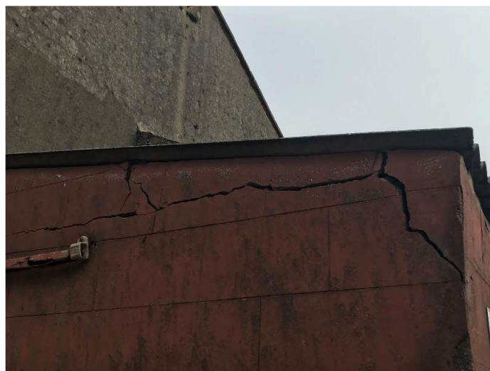
Figure 3.5 – Cracking at purlin bearings
