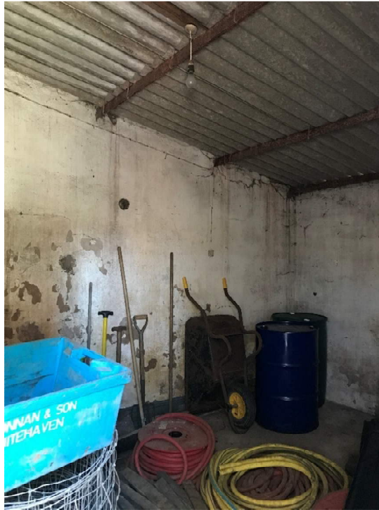
Figure 3.6 – Water staining and cracking to internal wall
