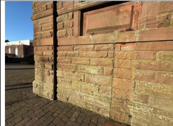
General Masonry Pointing – Deleterious mortar pointing.
