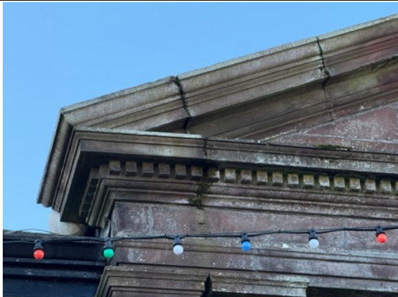
Stonework Repairs – Essential pointing repairs required to portico.
