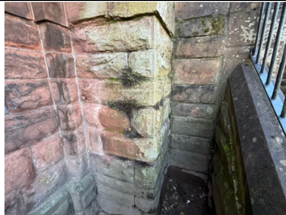
Stonework Cleaning – Sandstone façade greening with moss and algae.
