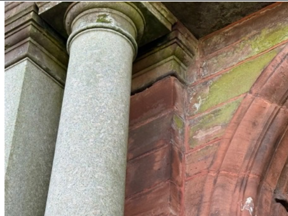
Stonework Repairs – Essential pointing repairs required to portico and sandstone façade.
