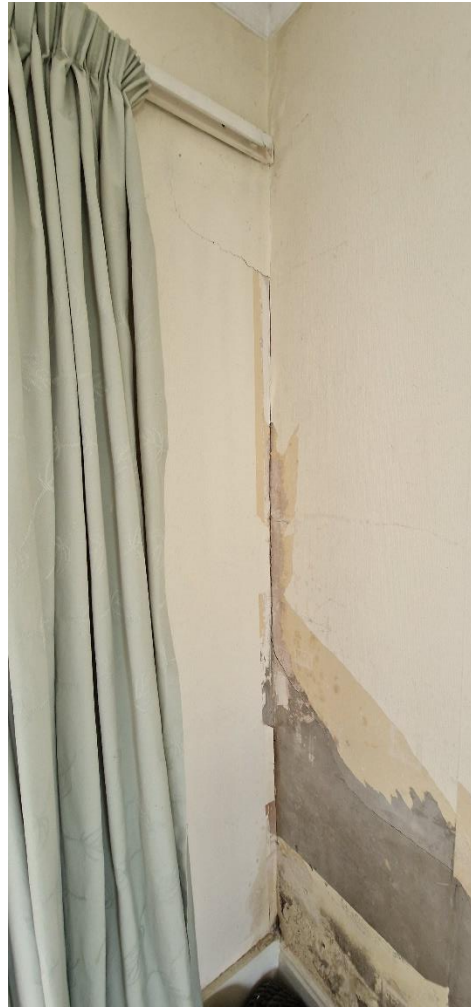
Photo 5 - Right Reception - Cracking to Rear Right
