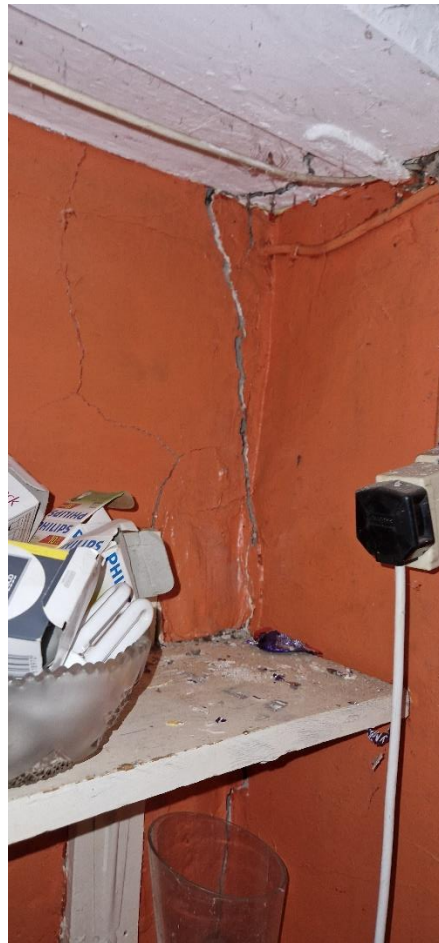
Photo 7 - Cracking in Cupboard
