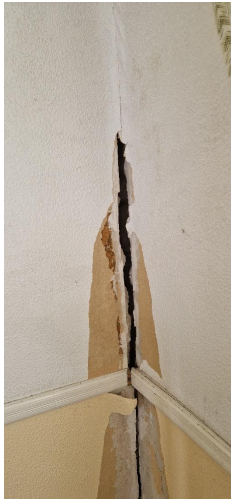
Photo 9 - Hall - Vertical Crack to Left Side at Rear
