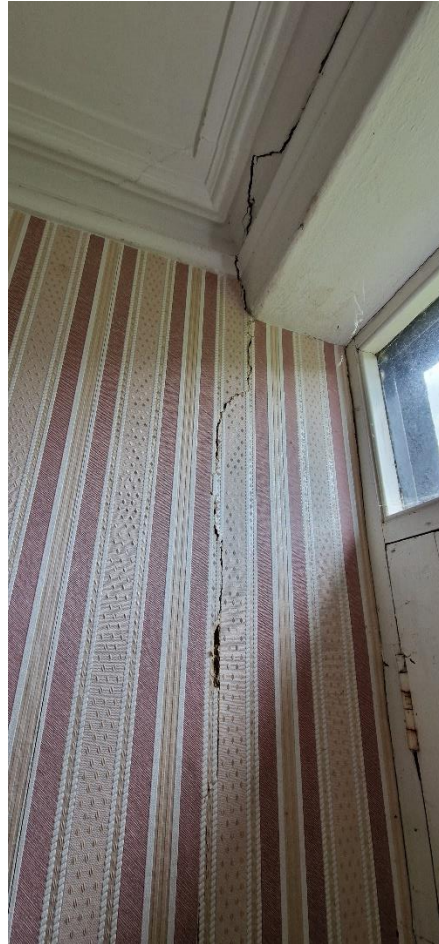
Photo 3 – Cracking Around Front Door
