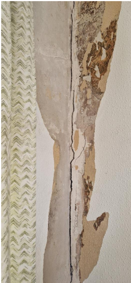
Photo 8 - Hall - Vertical Crack to Right Side at Rear
