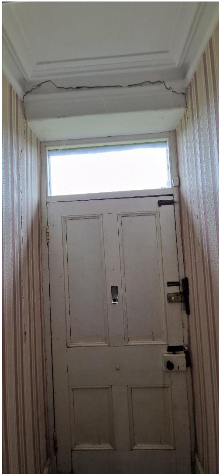
Photo 2 - Cracking Around Front Door
