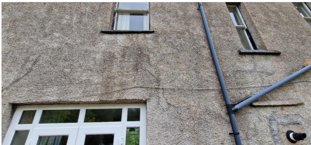
Photo 11 - Rear Elevation - Sporadic Cracking
