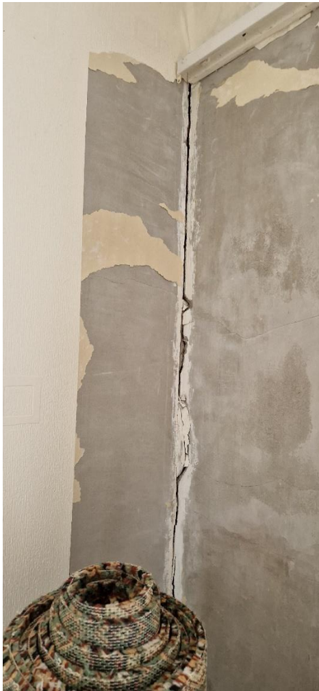
Photo 4 - Right Reception - Vertical Cracking to Rear Left
