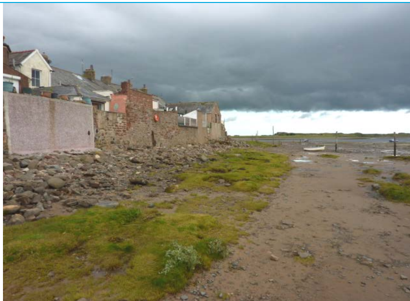
Figure 9-2: Masonry wall protecting Ravenglass properties (top). Man-made coastline defence near Monk Moors to the south of the Esk River Mouth (middle). Ravenglass flood gate (bottom).
